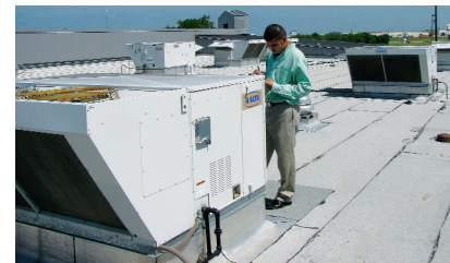
EMA Graduate Engineer Javier Garcia checks AC units for underperforming controls during a recent commissioning project.
