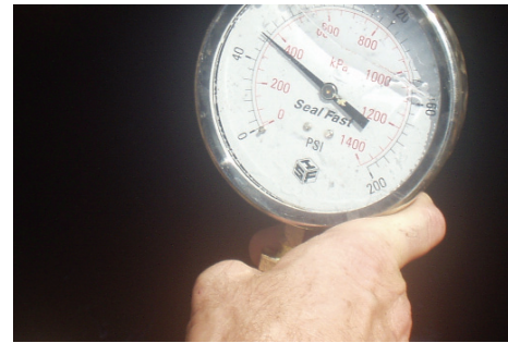
During the commissioning process instrumentation is used to gather data to evaluate systems performance.
