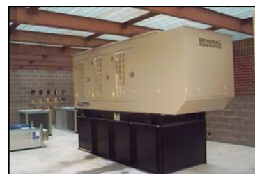
Figure 2. Typical Generator Set
