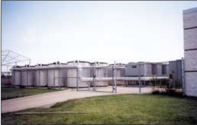
Designed by Estes, McClure & Associates, the central thermal storage plant for the Plano school complex works at night to create ice which is stored in the tanks at left. During the day, the ice is melted to provide chilled water for cooling the complexes three campuses.
